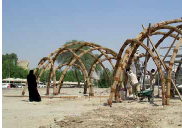
Bakheeta Humaid Dubaila Dhahi Al Mansoori, student from the Zayed University volunteering for the project's construction © Sandra Piesik.
