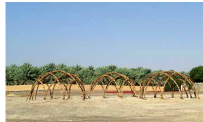
Early construction stage of The Food Shelter next to Al Ain Oasis © Sandra Piesik.
